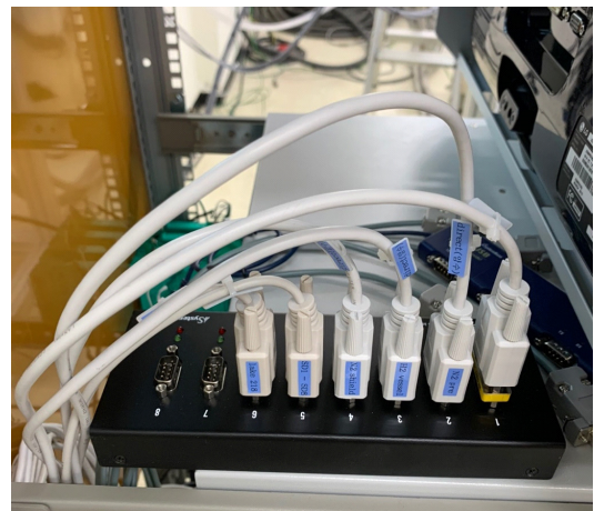
Fig. 7. Cables connected RS-232 and RS-485 converters
